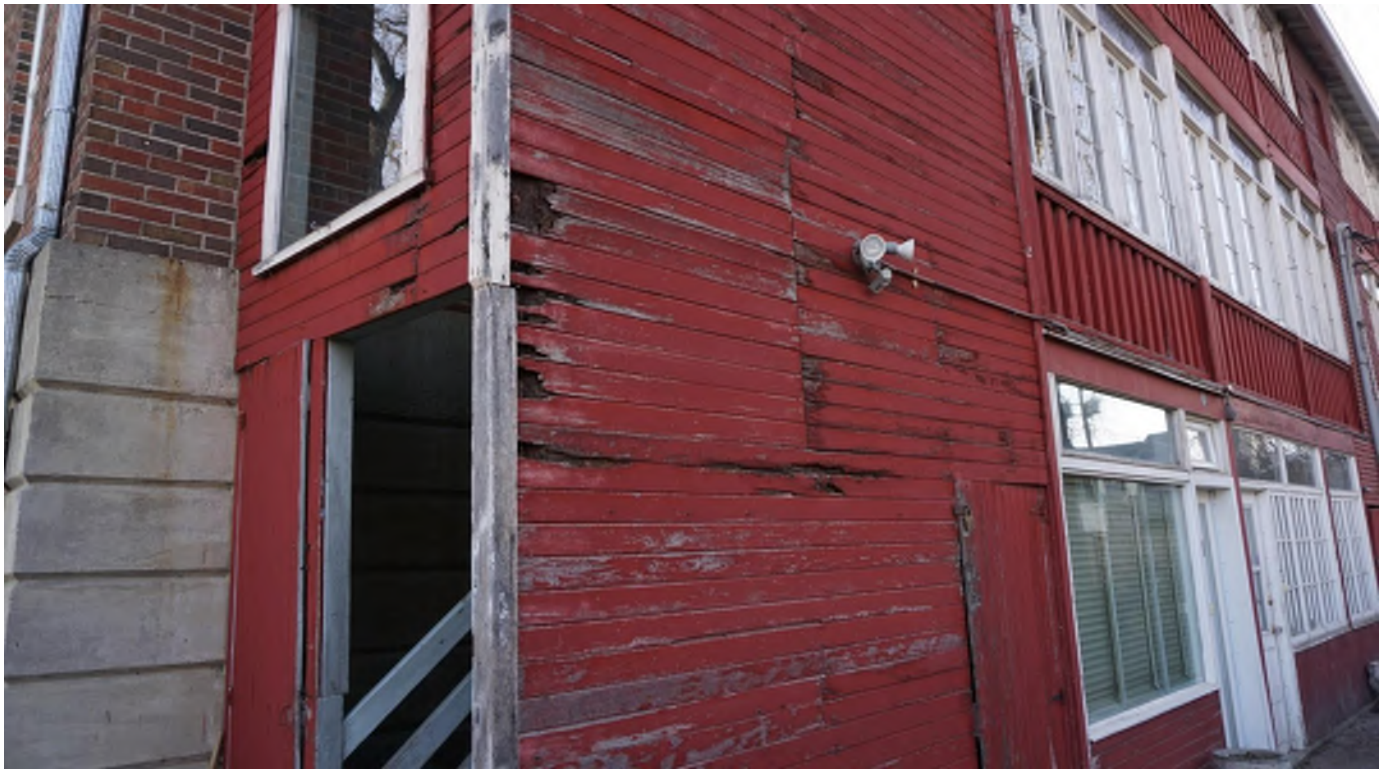
Figure 18 - Example of extensive deterioration of the wood siding.
