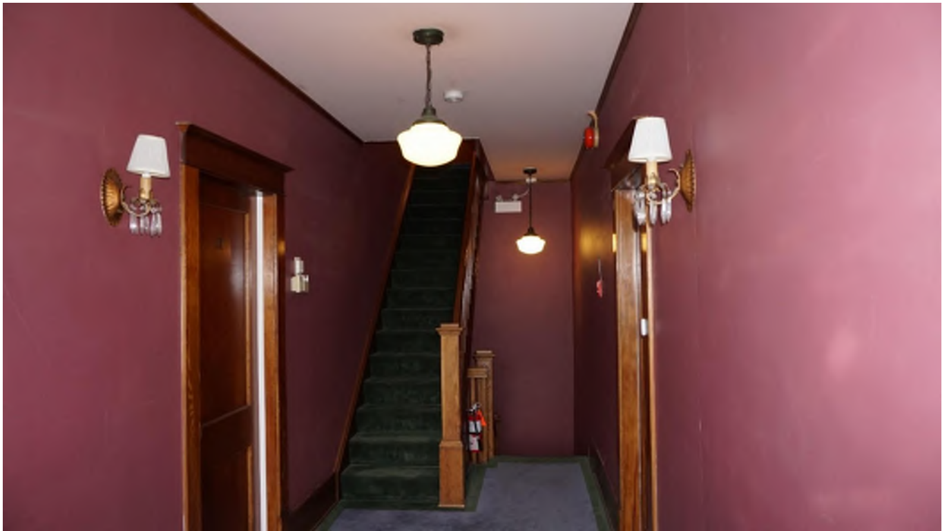
Figure 25 - Pendant and wall mounted hallway and stairwell fixtures.
