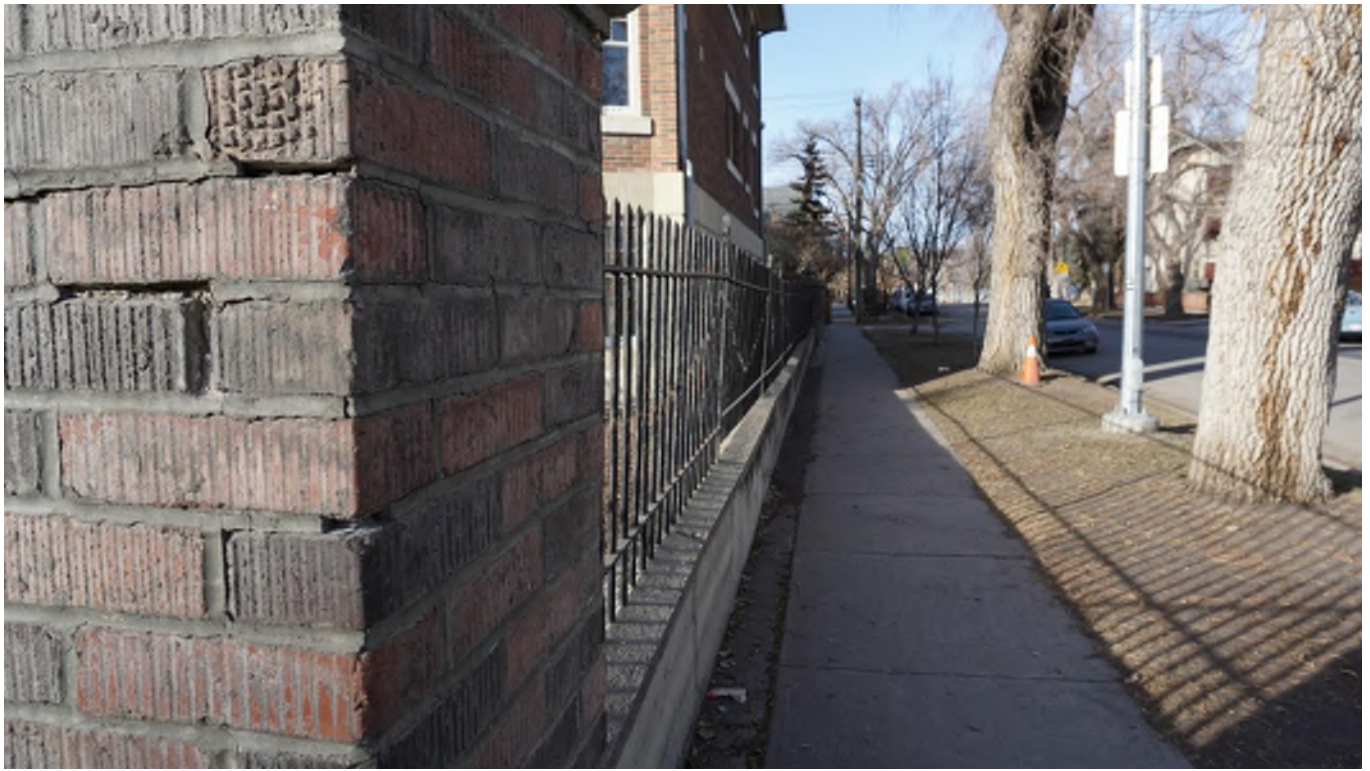
Figure 67 - Some leaning of the metal fence.
