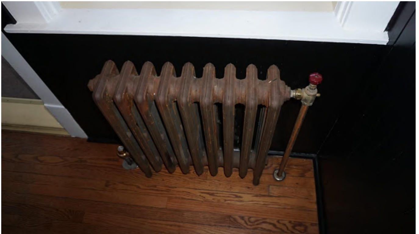
Figure 33 - In-suite cast iron radiator.
