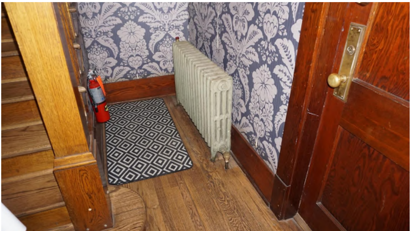
Figure 34 - Common area cast iron radiator.
