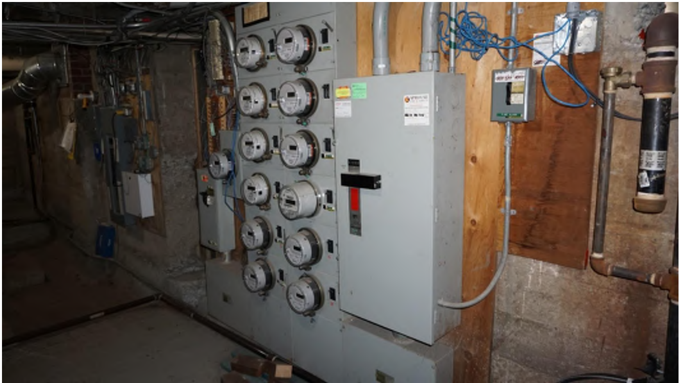
Figure 27 - Power distribution equipment in the basement.
