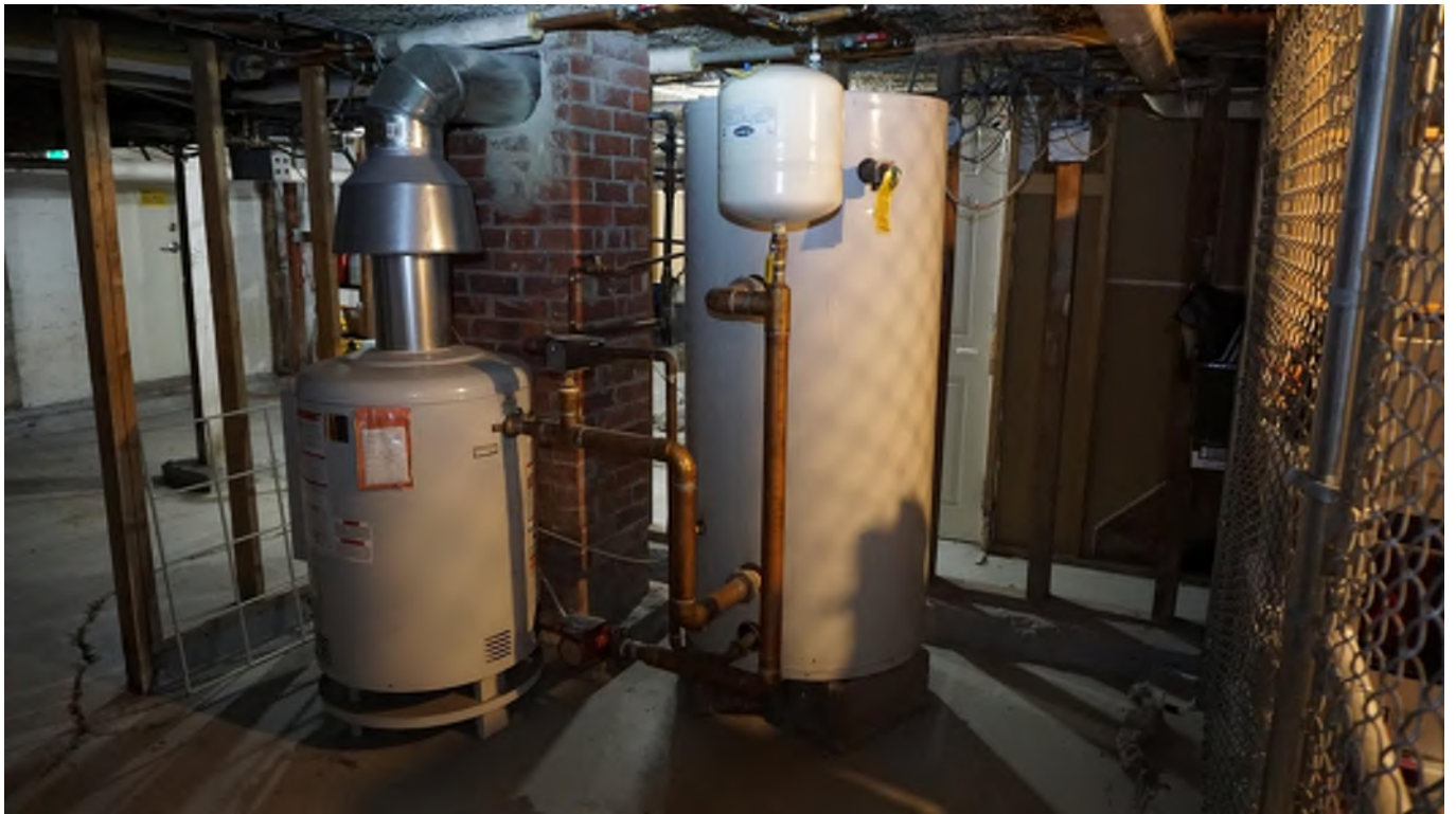
Figure 30 - AO Smith hot water supply boiler, storage tank and expansion tank.
