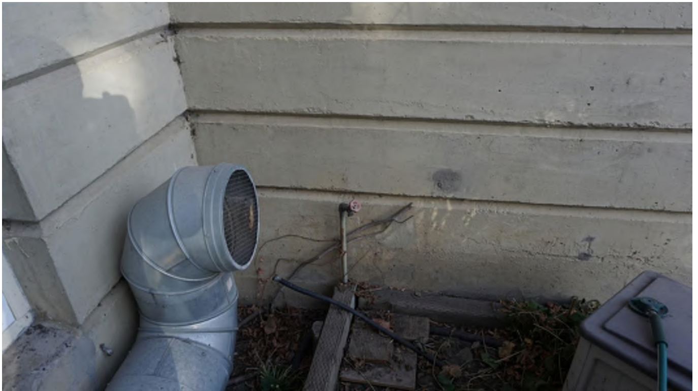
Figure 37 - Exterior hose bibb.
