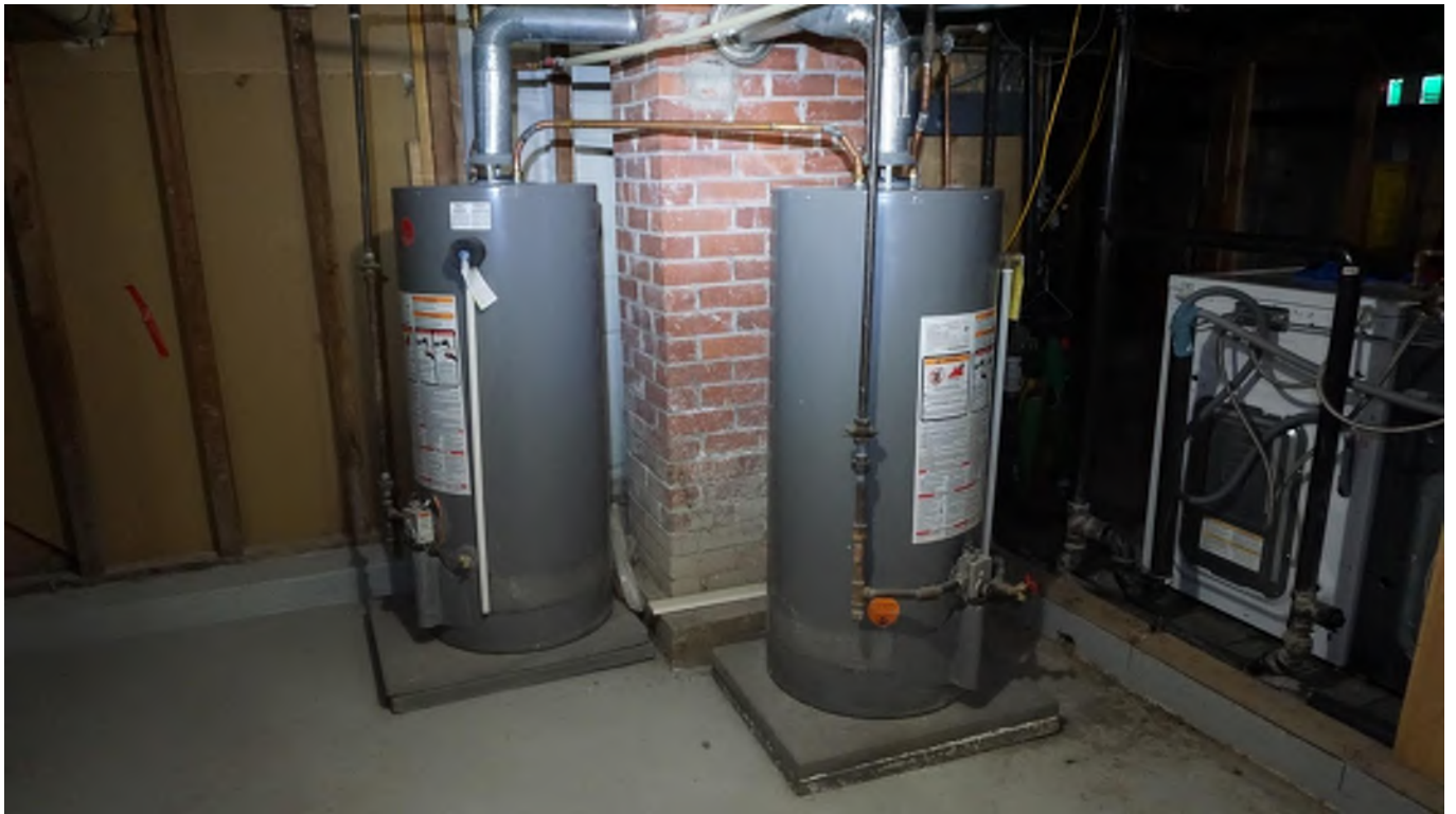
Figure 32 - Rheem domestic hot water heaters.
