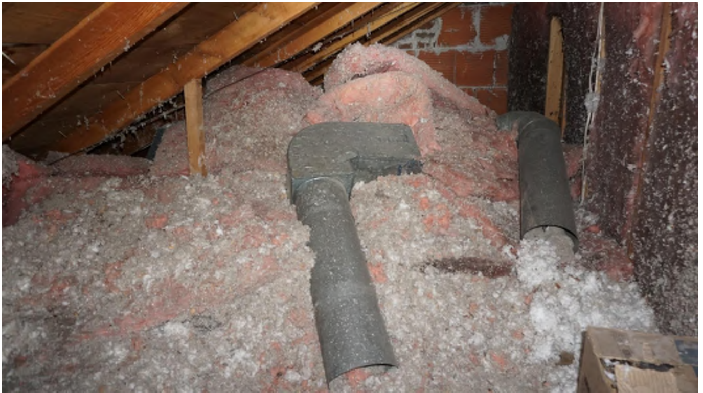
Figure 4 - Example of disturbed insulation and surplus ducting.
