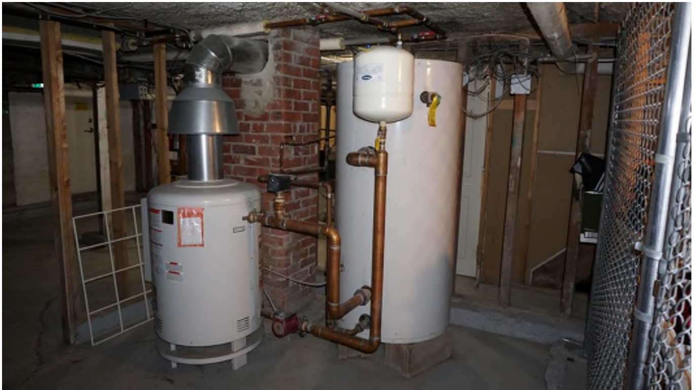
Figure 31 - Copper to galvanized piping along basement ceiling.
