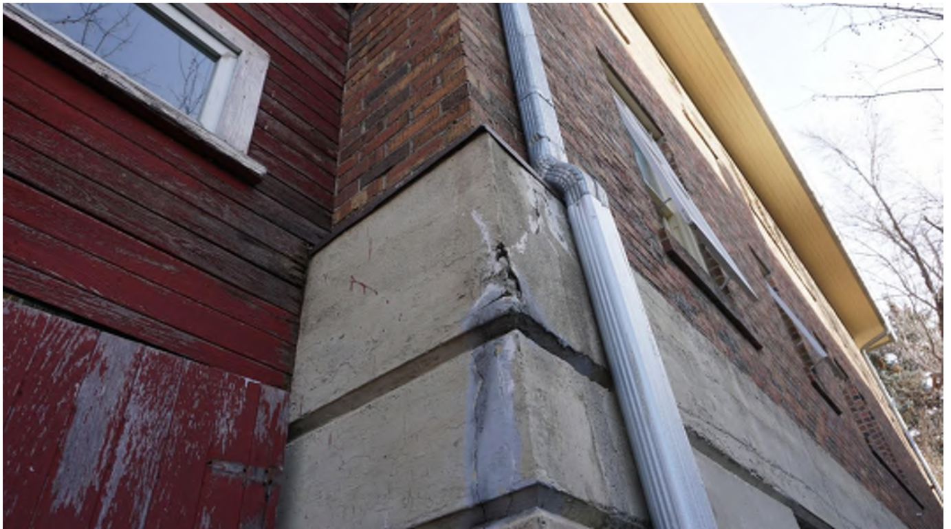
Figure 1 - Example of decorative features of the foundation wall and spawl damage due to previous downspout failure.
