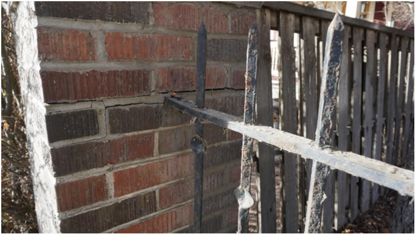
Figure 68 - Example of metal corrosion and mortar cracking typical on the fence.
