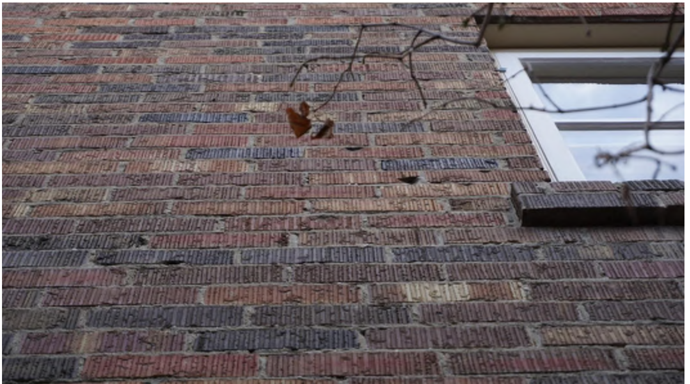
Figure 7 - Example of fluted style clay bricks showing some brick and mortar damage.
