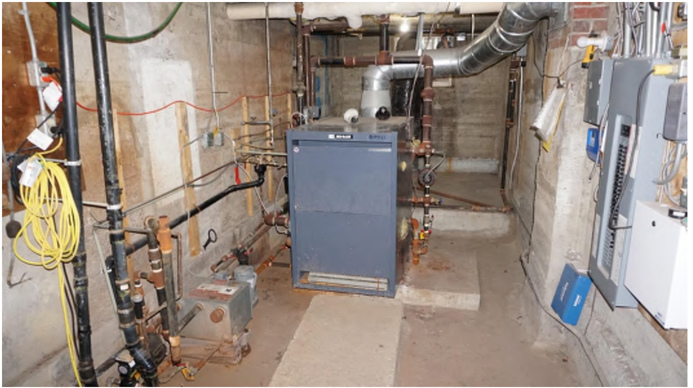
Figure 29 - Weil-McLain steam boiler.
