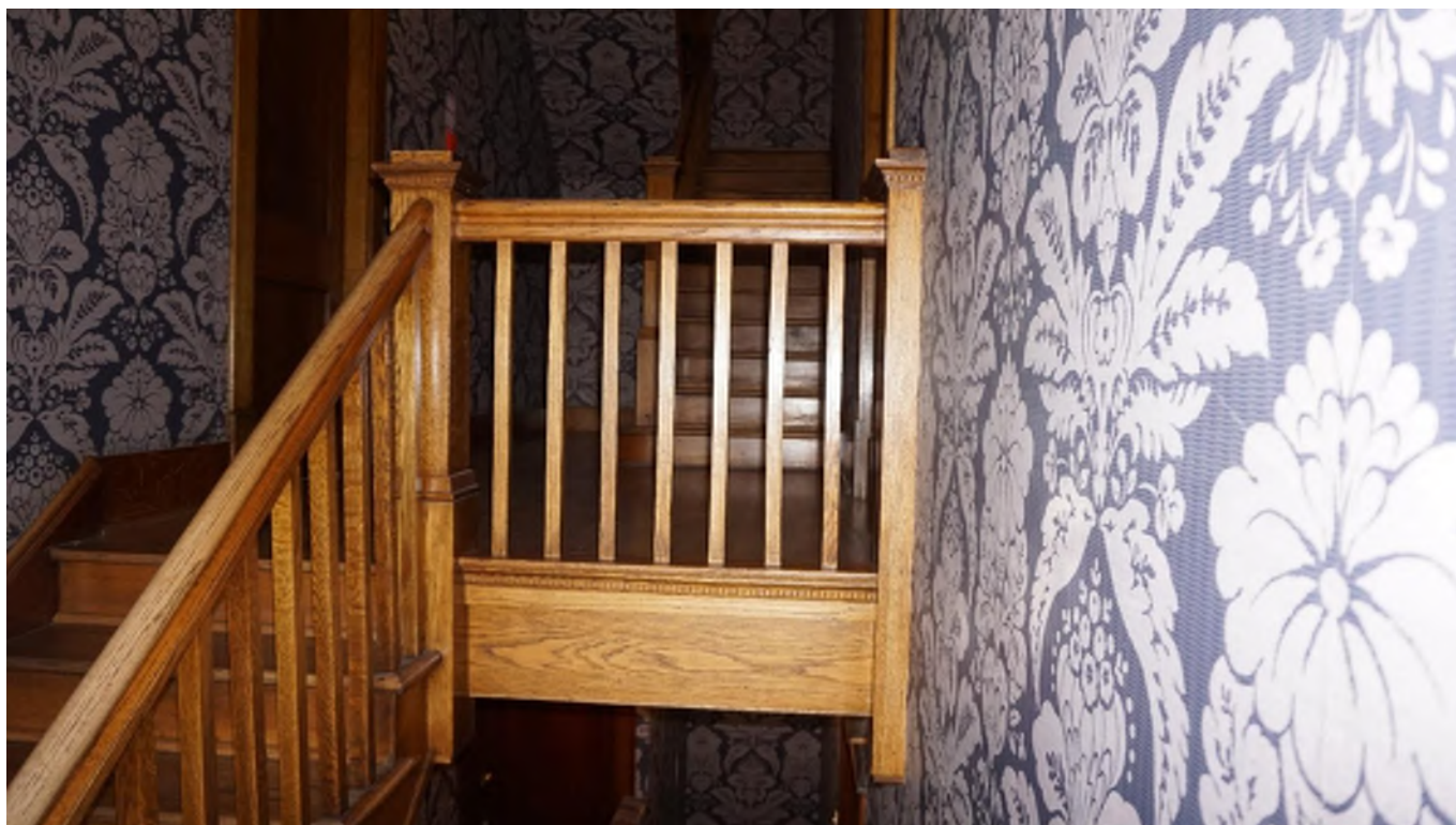
Figure 52 - Stairwell posts and rails in Building 904.
