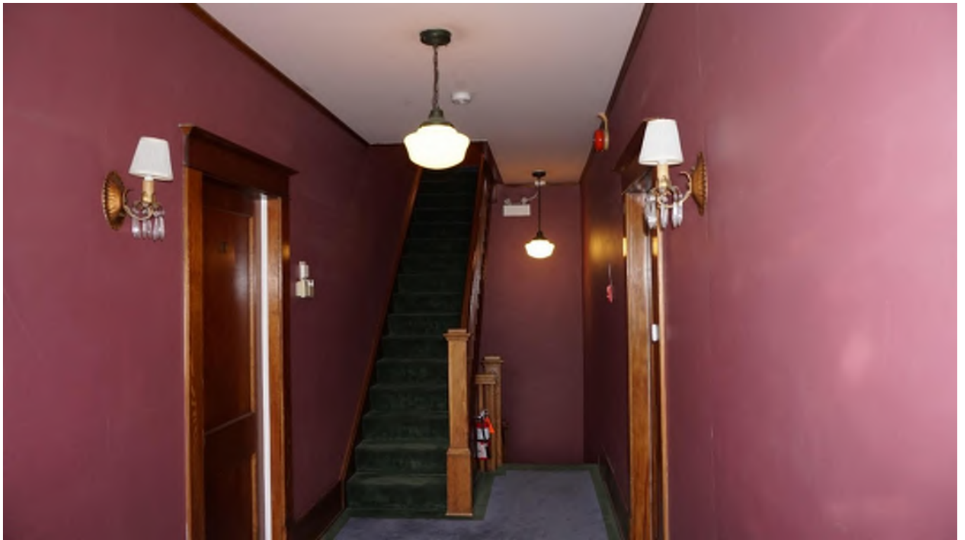
Figure 43 - Shows manual pull station, bell and emergency lighting.
