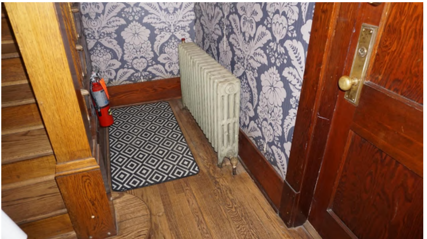
Figure 42 - 5lb fire extinguisher.
