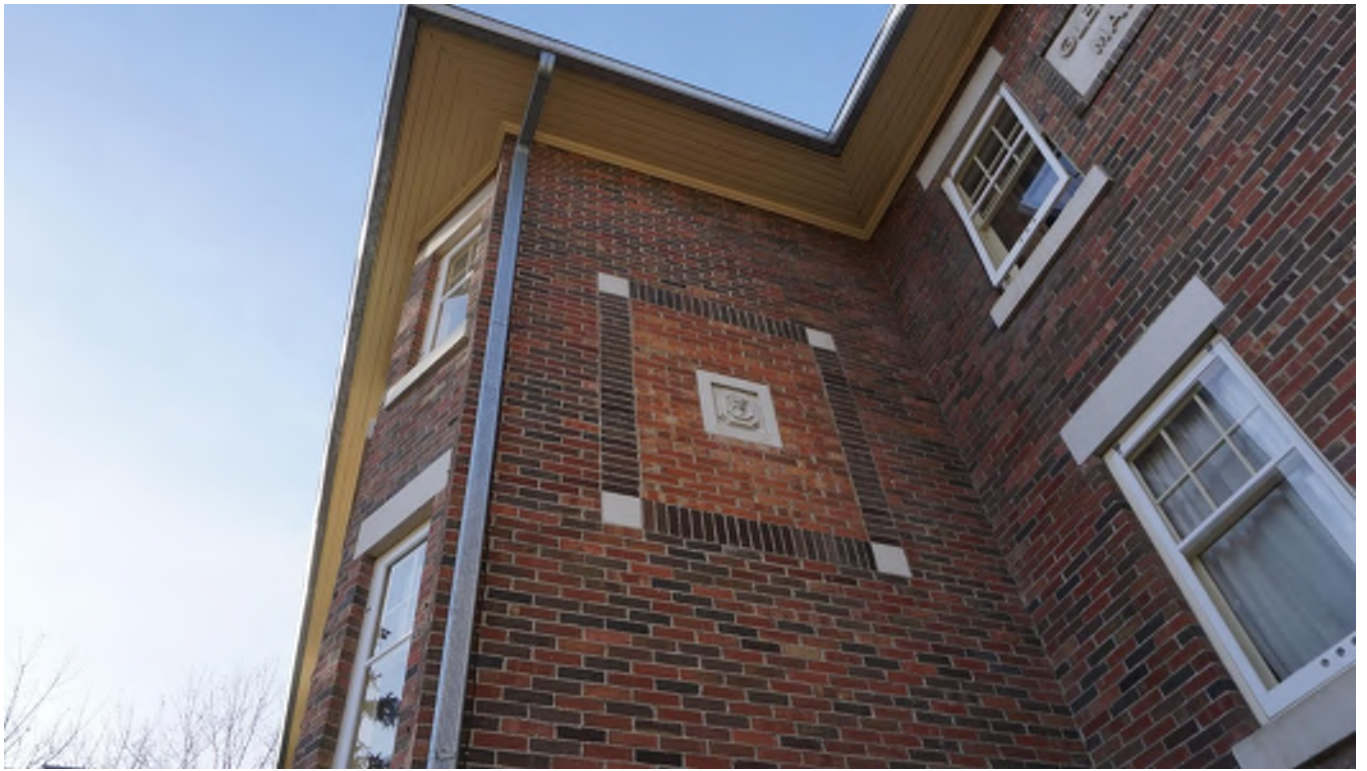
Figure 19 - Example of painted wood soffit boards.
