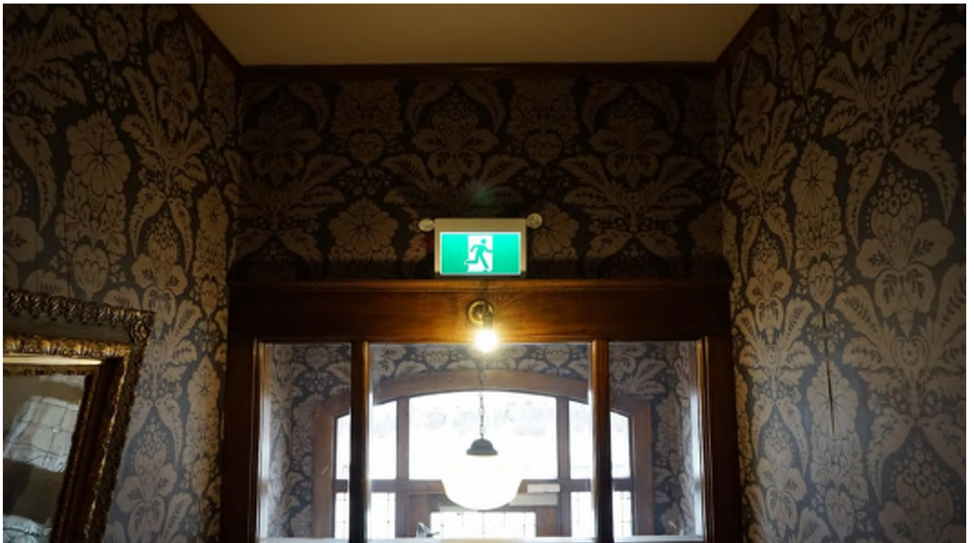
Figure 44 - Exit signage and emergency lighting combo.
