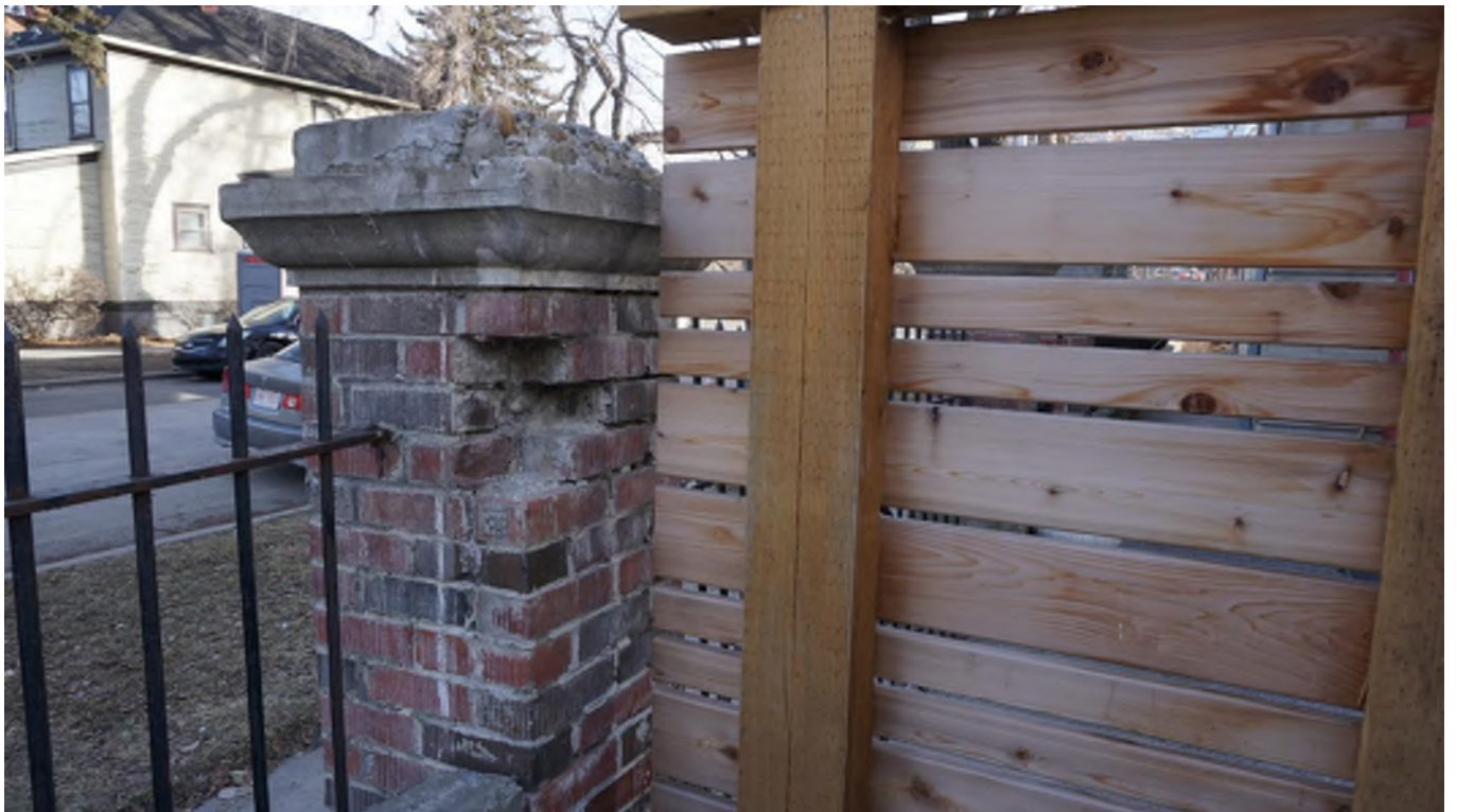
Figure 66 - Significant deterioration of a column at the northeast corner.
